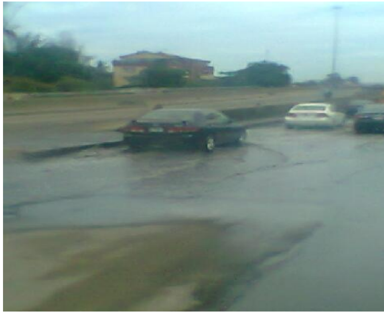
FIGURE C: BAD ROAD CONDITION AT THE BRIDGE DIVERSION ALONG CREEK ROAD
