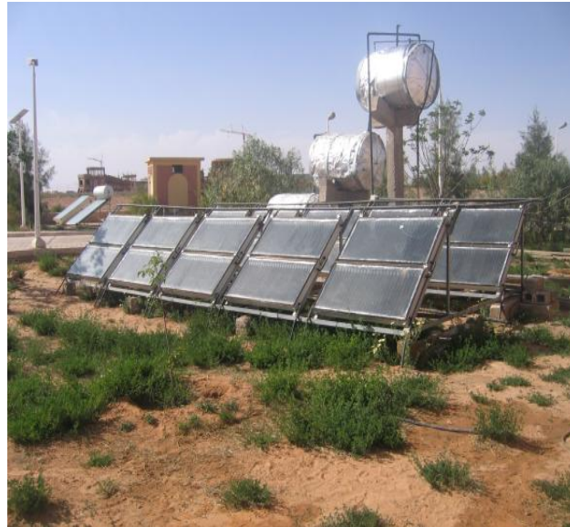
Figure 3. Collective installation of solar heater in Algerian Sahara
