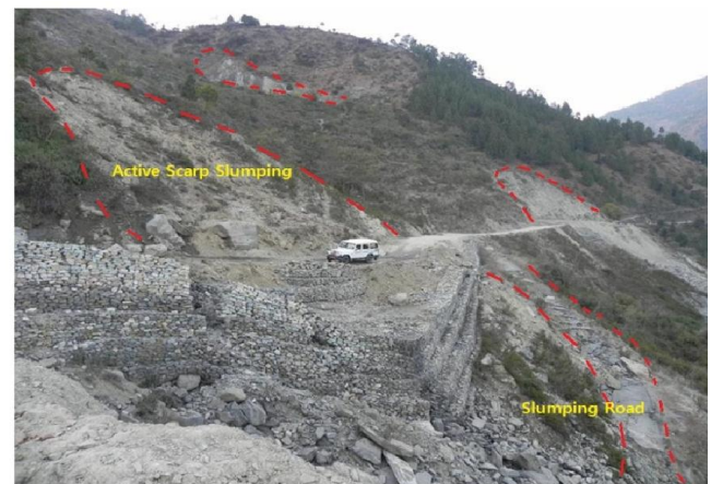
Plate 3. Slumping of motorable road
