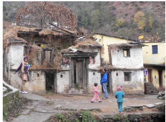
Plate 4. Damaging houses due to slumping
