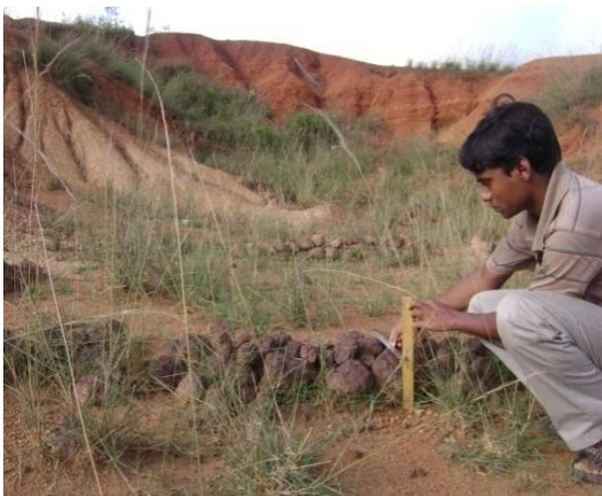
Figure 5. Typical porous check dams constructed with local bolder for sediment trapping and reducing runoff. (A) Sept, 2009, and (B) Oct, 2010
